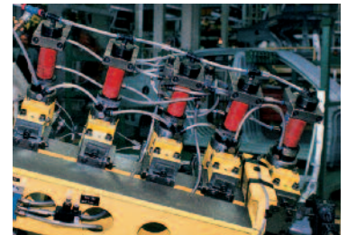
Stamping units placed in line
